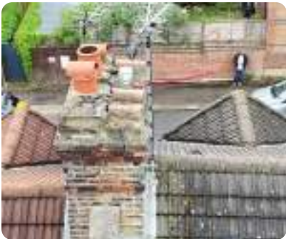
Photo 7 View of the chimney stack from the roof; visible deterioration of the mortar and missing pots at the top of the stack.
