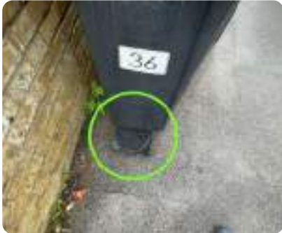
Photo 134 Water meter valve box.
