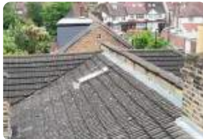
Photo 5 Main roof concrete interlocking tiles generally appear to be in an adequate condition but spalling render on valleys requires repair. Some mild deflection identified on the rear roof junction
