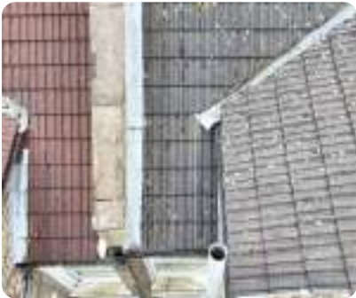
Photo 16 Main roof concrete interlocking tiles generally appear to be in an adequate condition but spalling render on valleys requires repair.
