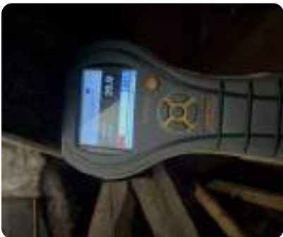
Photo 116 High Moisture Readings and Locations - Loft Valley rafter.
