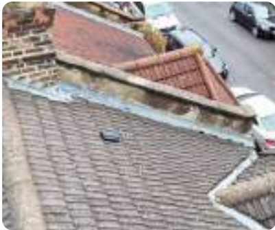
Photo 11 Main roof concrete interlocking tiles generally appear to be in an adequate condition but spalling render on valleys requires repair.
