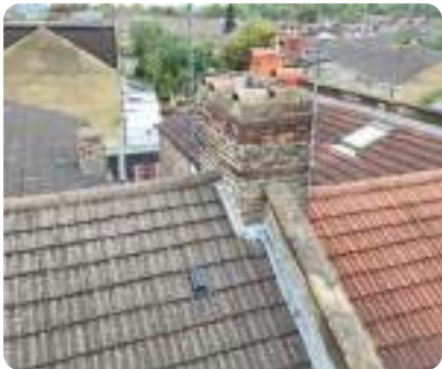
Photo 26 Main roof concrete interlocking tiles generally appear to be in an adequate condition but spalling render on valleys requires repair.
