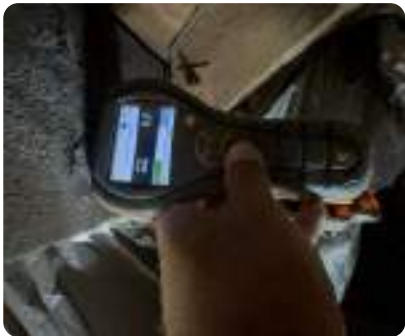
Photo 112 Roof void showing high moisture reading of 9.7%, indicating potential damp issues.
