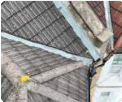
Photo 30 Main roof concrete interlocking tiles generally appear to be in an adequate condition but spalling render on valleys requires repair.
