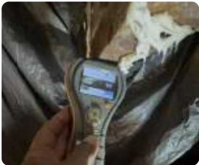
Photo 115 Roof void showing moisture meter reading of 9.5%, indicating potential moisture presence.
