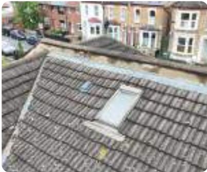
Photo 18 Main roof concrete interlocking tiles generally appear to be in an adequate condition but spalling render on valleys requires repair.
