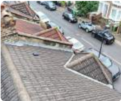
Photo 9 Main roof concrete interlocking tiles generally appear to be in an adequate condition but spalling render on valleys requires repair.
