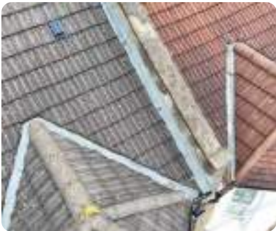
Photo 25 Main roof concrete interlocking tiles generally appear to be in an adequate condition but spalling render on valleys requires repair.
