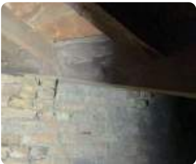
Photo 117 High Moisture Readings and Locations
