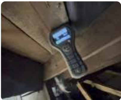
Photo 118 High Moisture Readings and Locations
