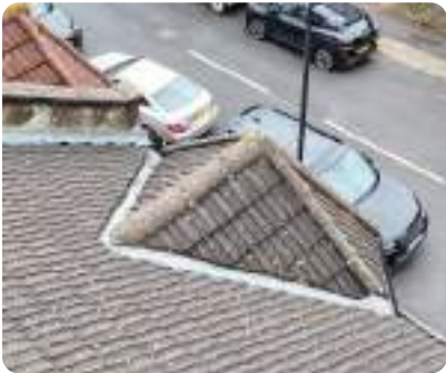
Photo 10 Main roof concrete interlocking tiles generally appear to be in an adequate condition but spalling render on valleys requires repair.
