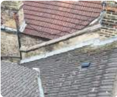
Photo 12 Main roof concrete interlocking tiles generally appear to be in an adequate condition but spalling render on valleys requires repair.
