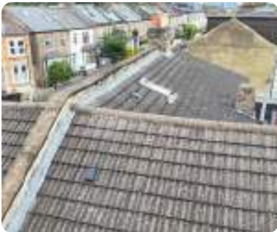
Photo 27 Main roof concrete interlocking tiles generally appear to be in an adequate condition but spalling render on valleys requires repair.
