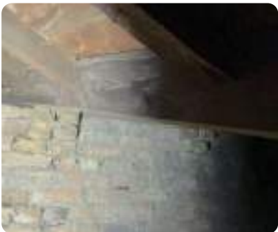
Photo 117 High Moisture Readings and Locations
