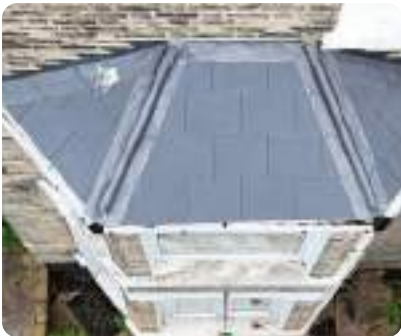
Photo 31 Roof covering over the bay window; the flashing appears to have damage with potential water ingress at the join.
