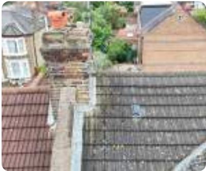
Photo 17 Main roof concrete interlocking tiles generally appear to be in an adequate condition but spalling render on valleys requires repair.
