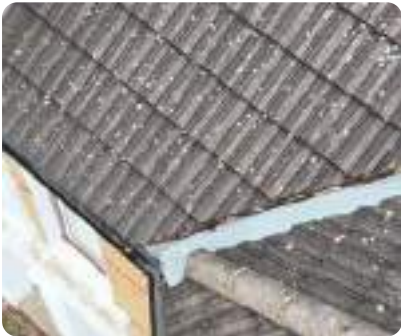
Photo 28 Main roof concrete interlocking tiles generally appear to be in an adequate condition but spalling render on valleys requires repair.
