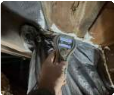
Photo 114 Roof void with moisture meter readings indicating 8.4% moisture content; evidence of possible dampness present.
