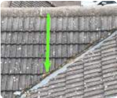
Photo 13 Spalling render to the valley rafter. Possible cause of leak into the receptacle in roof space below.
