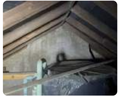
Photo 97 Roof void showing timber rafters and water-stained wall; evidence of possible dampness indicated by discoloration on the wall.
