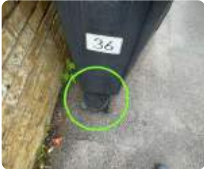
Photo 134 Water meter valve box.
