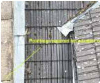
Photo 14 Main roof concrete interlocking tiles generally appear to be in an adequate condition but spalling render on valleys requires repair.
