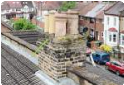
Photo 4 Rear chimney stack on the main roof but some wear on the flaunching.
