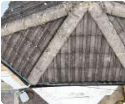
Photo 29 Main roof concrete interlocking tiles generally appear to be in an adequate condition but spalling render on valleys requires repair.
