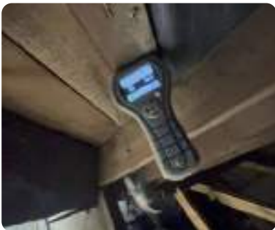
Photo 118 High Moisture Readings and Locations
