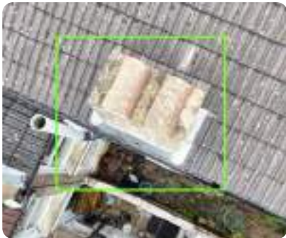
Photo 15 In the room below this chimney, there is salt contamination on the chimney breast.
